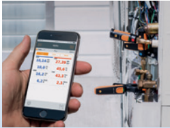
Efficient adjustment of refrigeration systems
